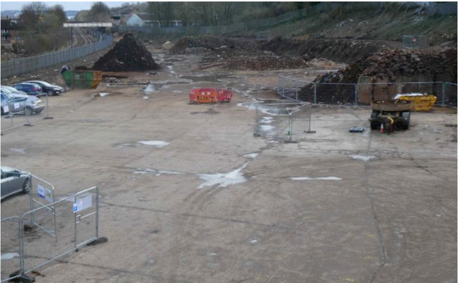
A view west from the road bridge that crosses the site shows clearance work in progress on 28 March 2024.
